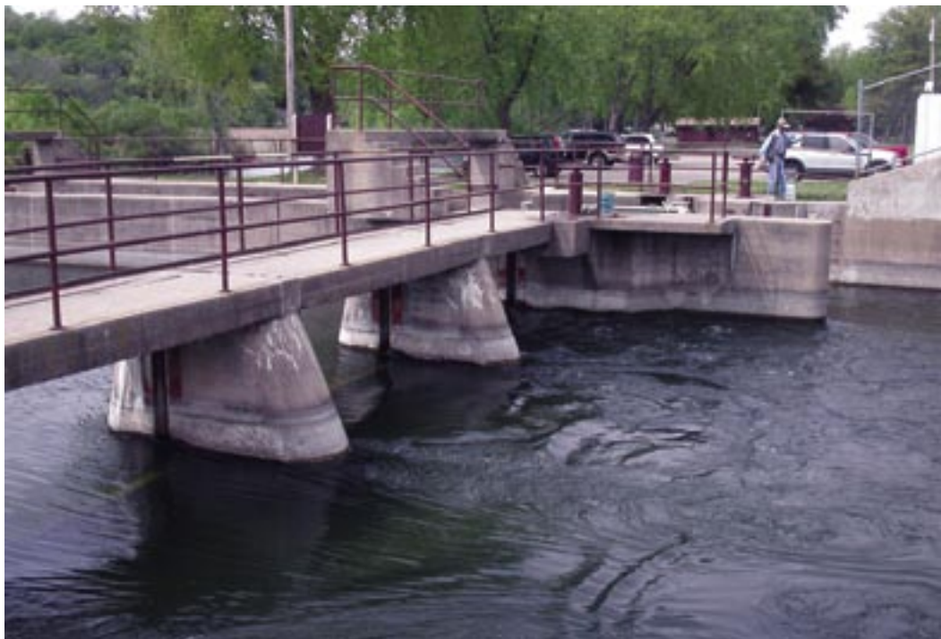
Figure 7. Lake Waubesa outlet structure. Note the stoplogs below the walkway barely produce a ripple in the water surface. Photo: B. Halverson, Baird & Associates.
